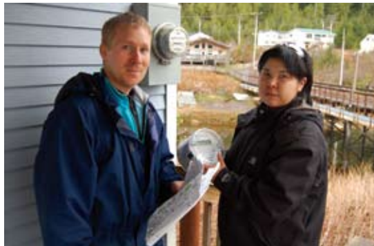
Dr Michael Wrinch PEng (left) and electrician Adrienne Nisyok (right) inspect and install the first smart electrical meter.
